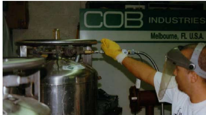
Connecting to the liquid nitrogen and starting the freeze.
